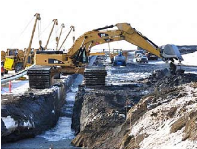
Price Gregory ENI Pipeline Project side booms preparing to place pipe in ditch. Nanuq Inc. is performing the ditch excavation.
