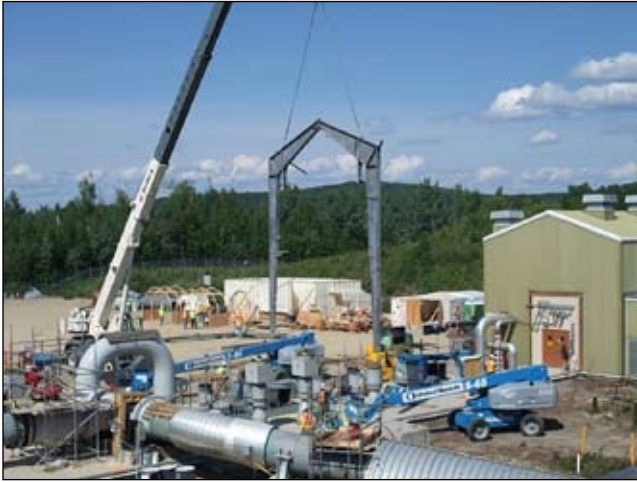
The last structure being removed by CASI Employees from the manifold building at Pump Station 8.
