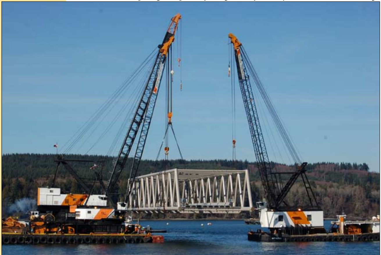
General Construction placing a ramp on the floating section of the newly renovated Hood Canal Bridge.
