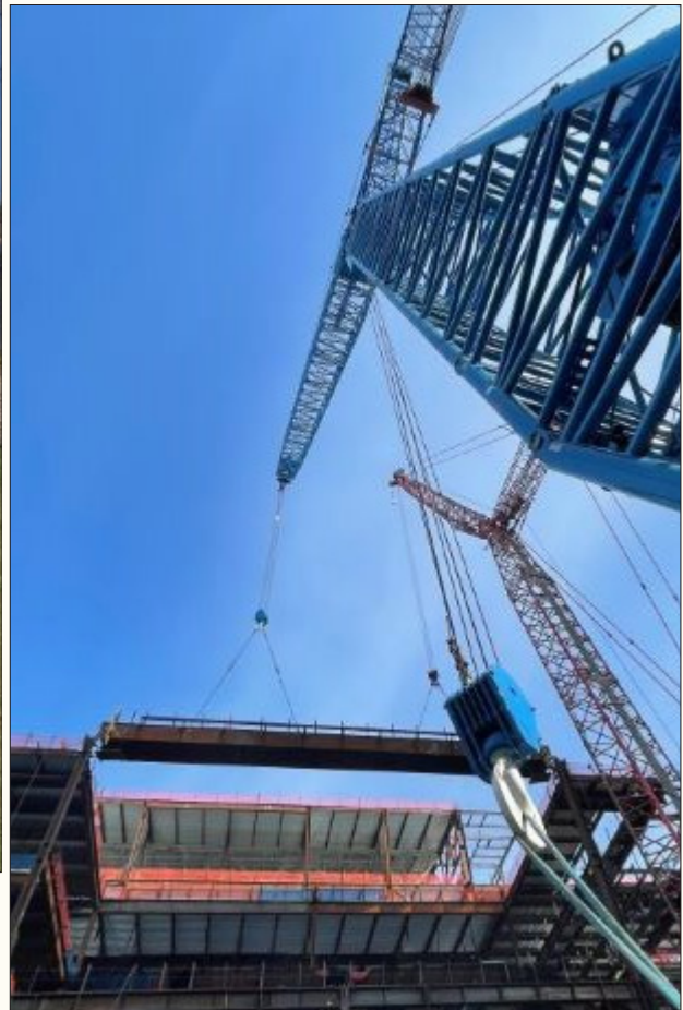
Below: Adam Wojcik of Mayfield Hoisting on the Washington State Convention Center site.
