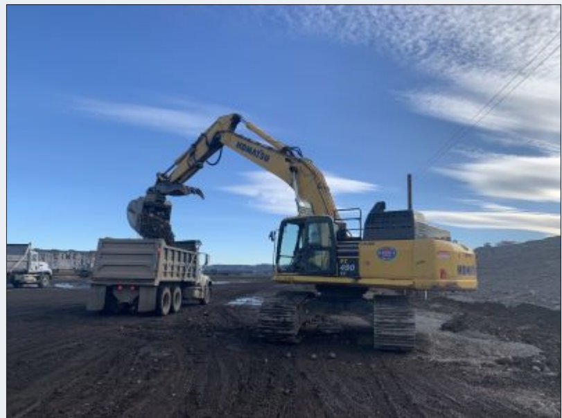
Above: Cory Anderson working for Scarsella Brothers on the Hwy 41 project in Northern Idaho.
