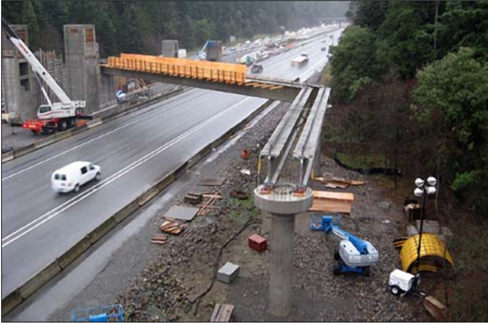
In mid-February, the state Department of Transportation shut down all northbound lanes of I-5 to install two pre-cast concrete girders over the freeway that will become a pedestrian walkway connecting the new Mountlake Terrace Freeway Station with the parking garage. (Photo & caption courtesy of Sound Transit)
