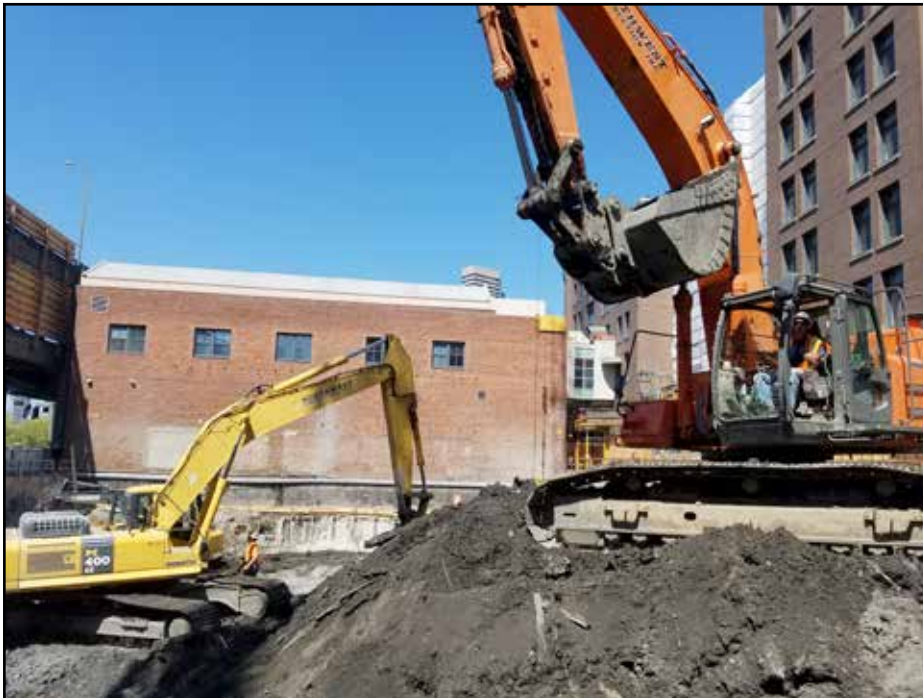
Laura Biesanz and Mike Wallace excavating for Northwest Construction on the Alaskan Way & S King St project for GLY
