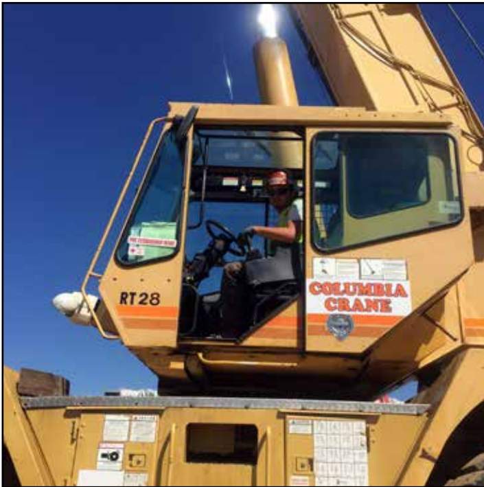
Apprentice Ryan Unger is running this hydraulic crane setting electrical boxes at the Yahoo project in Quincy.
