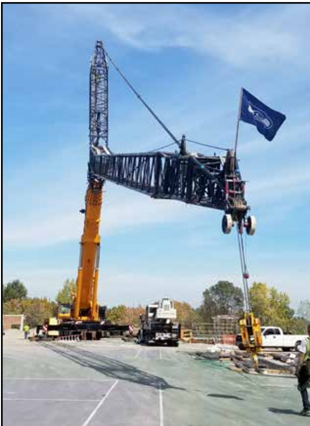
Doug Yuckert set up and ready to build another pair of Tower Cranes at the University of Washington.
