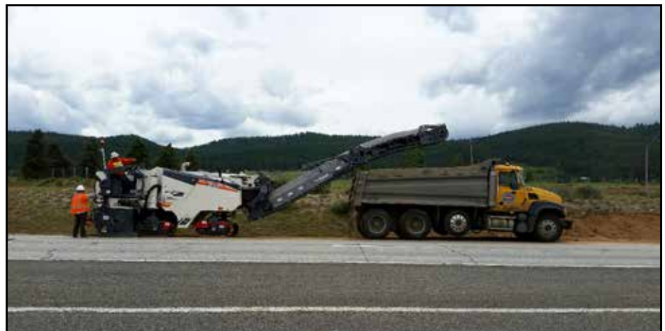
302 Member Dan Nisson operating the Roto-Mill machine with 302 Apprentice Kent Lester for Scarsella Bros on the I-90 Elk Heights project.
