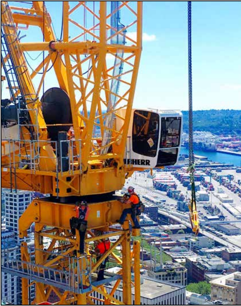
Northwest Tower Crane preparing to increase the elevation of Shawn Cook's crane at the 5th & Madison project for Sellen
