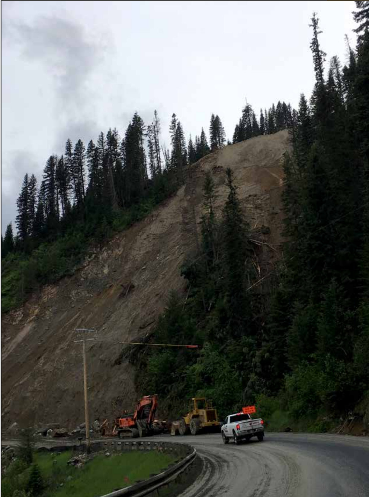
West Co. working on land slide at Elk City, Idaho
