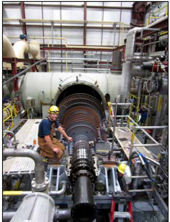
GVEA North Pole Power Plant Mechanics Virgil Bullard and Travis Kunkle during turbine repair.
