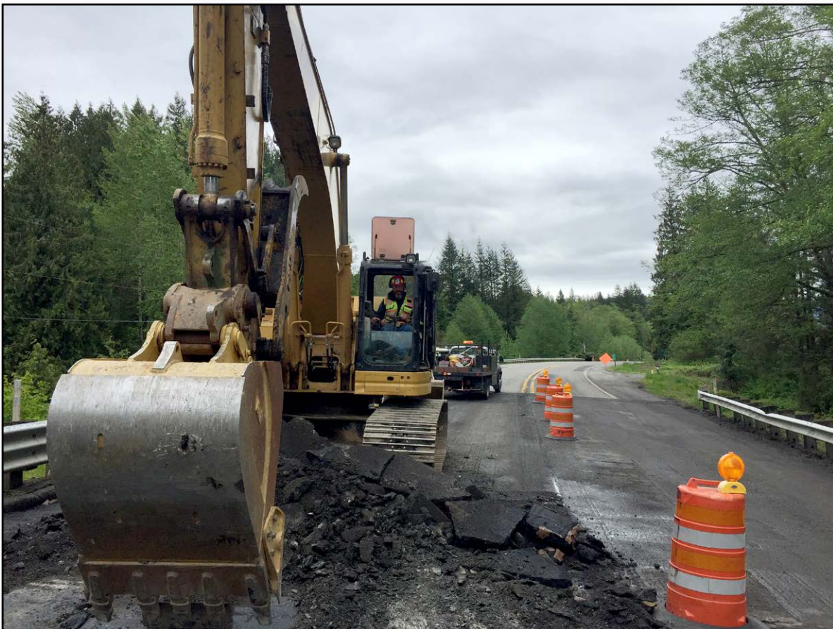
New member Wes Wallen working for Granite Construction in Hamilton on Highway 20
