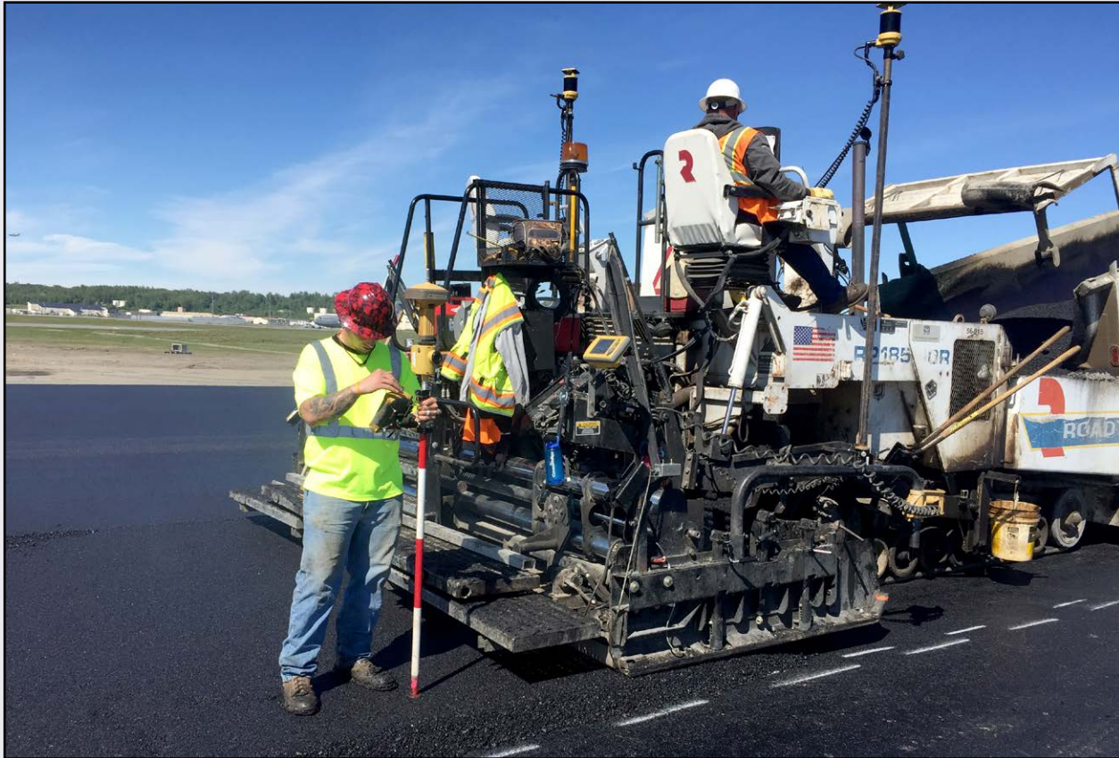
ASRC Civil Construction / Topside Paver Operator Dale Schram and Screed Operator A.J. DUBY paving on runway on JBER utilizing Topcon's 3D Millimeter GPS System
