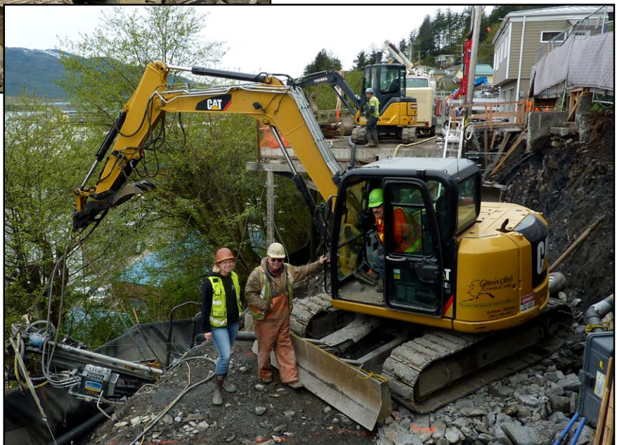
302 members Danielle Miller, Dave Cloudy, and Robert McDowell working for Glacier state Contractors in Ketchikan.
