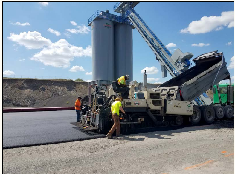
Tim Reeder, Leonard Adams, Terry Buckna, Shamrock Paving New Hot Plant set up.
