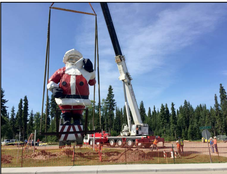
Precision Cranes - Owner Fred Kuykendall, Operator Jimmy Blevins, Tim Shorey Sr. and Kole Kuykendall
