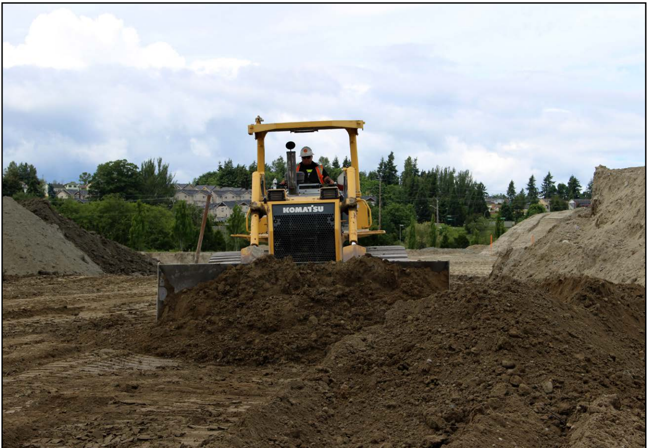
Apprentice Jaye Kesler Walls on the dozer at the Ellensburg Training Center.
