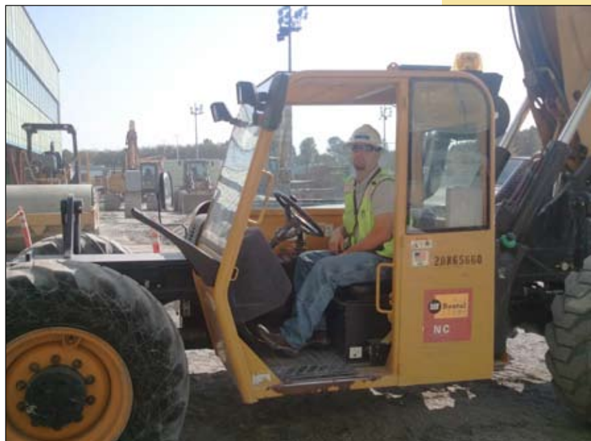
Josh Panas operating a forklift. Lifting building materials to the roof. Working for Skanska at The Boeing Everett Delivery Center project.
