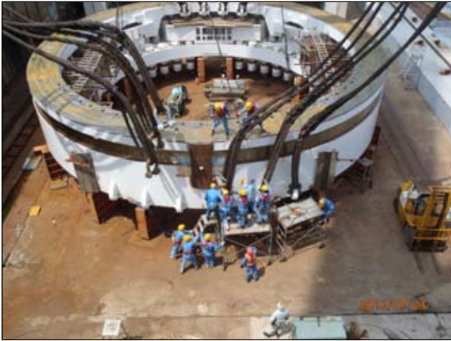
Cutter Head being built in Japan for the SR99 Deep Bore Tunnel
