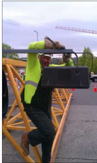
Forman - Scott (Barney) Hansen, working for Garner Const. Erecting another Tower Crane
