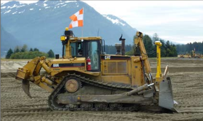
D8 Dozer with GPS at Juneau International Airport, Operator Apprentice Joel Wolf
