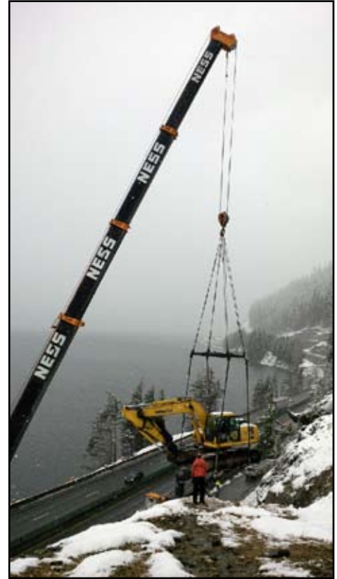
Ness Crane making a pick of KLB's excavator on the rock cliff I-90
