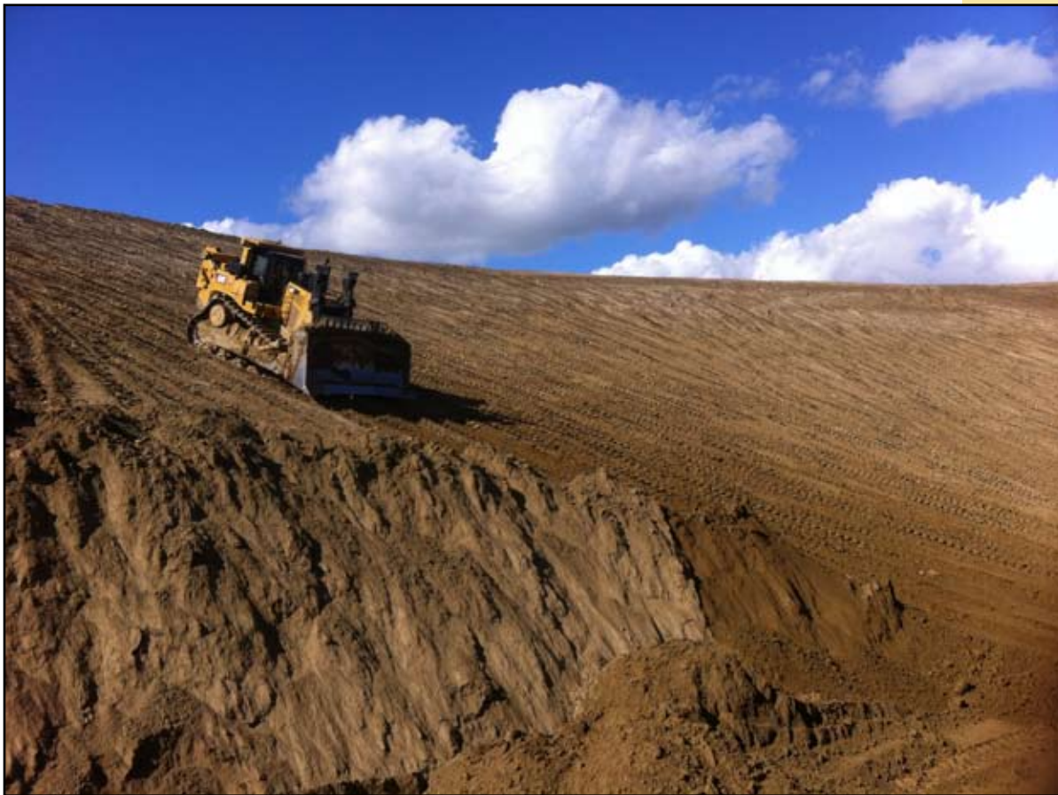
Apprentice Leo Kosmin at Browns Hill Quarry up in Fairbanks doing reclamation.
