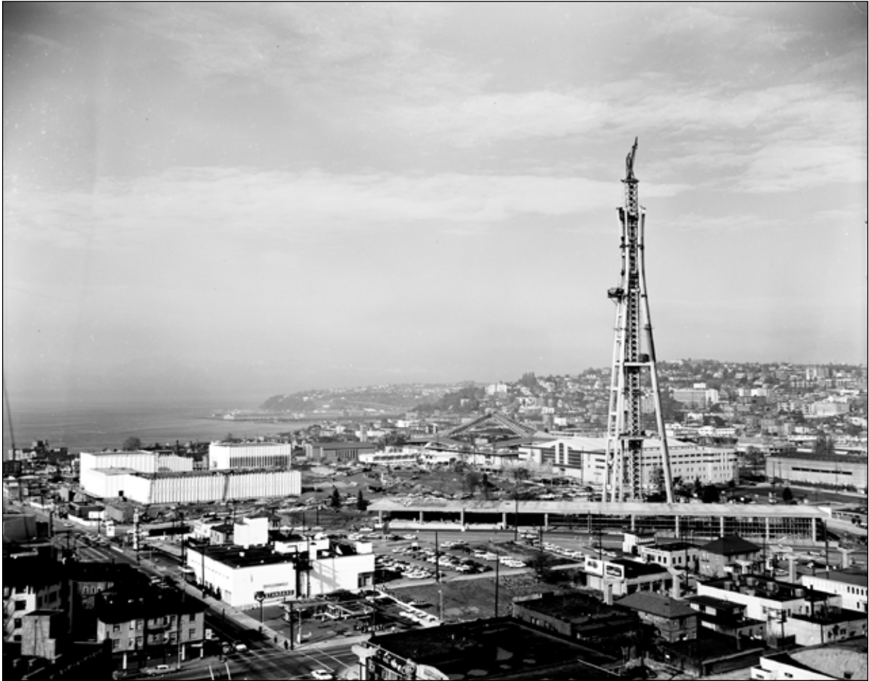
The Space Needle in Seattle is now 50 years old. Construction for the 1962 World's Fair
