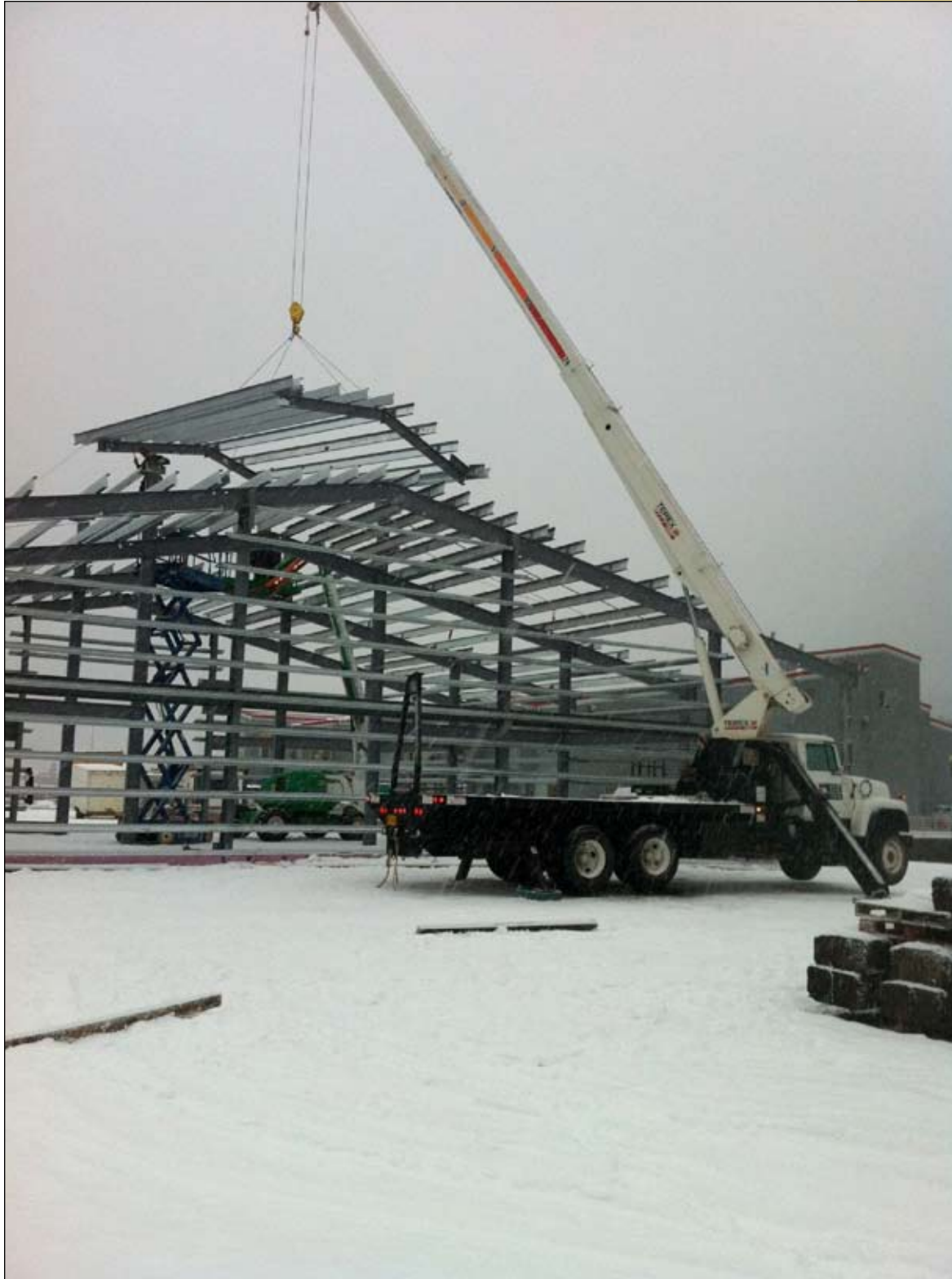
Nothing like hanging steel in the middle of winter. Eric Henricksen operating an 18 ton boom truck for North Pacific Steel Erectors on DIPAC's new warehouse in Juneau.
