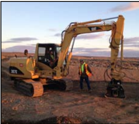
Left: Backhoe and Excavator instructor Dennis Grenninger giving first year apprentice Jeff Ancich some pointers on compacting with the hoe pack.
