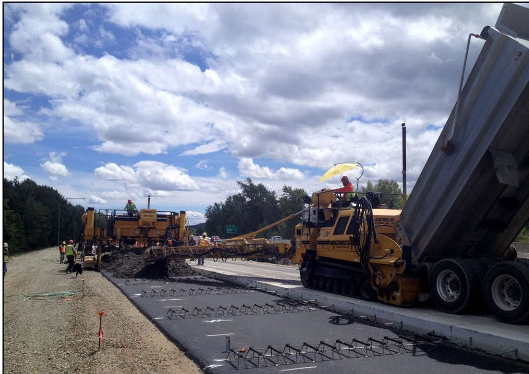
302 members on the concrete paving crew working for Gary Merlino making a new I-90 westbound truck lane in Cle Elum on the Mid Mountain Contractors project
