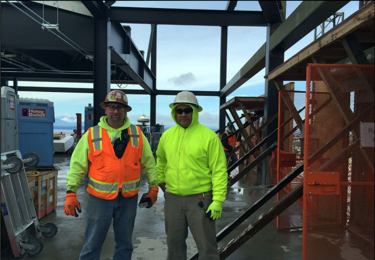
Fred Curry III and Vaoita Suitonu working for Sellen on Amazon's block 19 project
