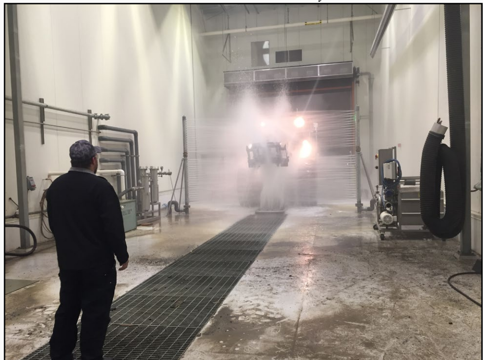
Wash Bay 3000 Gallons Per Minute
