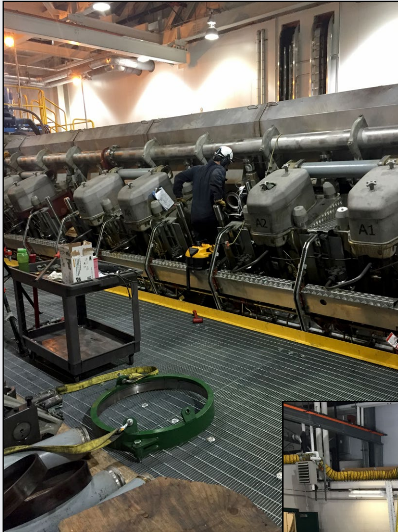
Maintenance Technician Dave Rodkey stepping into a cylinder bore. Matanuska Electric Association (MEA)
