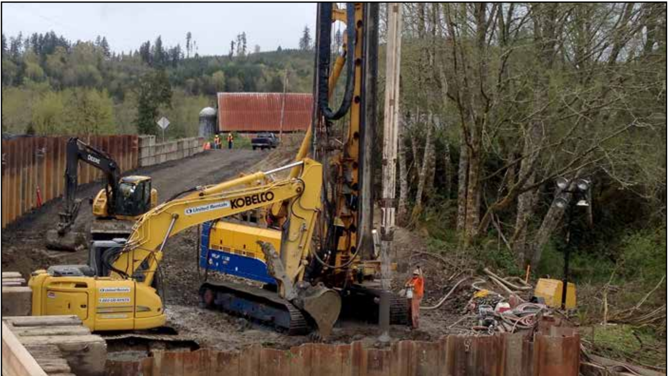
Gerard Creek Bridge Reinforcement Project in Oakville, WA Phillip Batiste (Local 115 Canada) driving pile - Mike Huffman (Local 302) on the excavator
