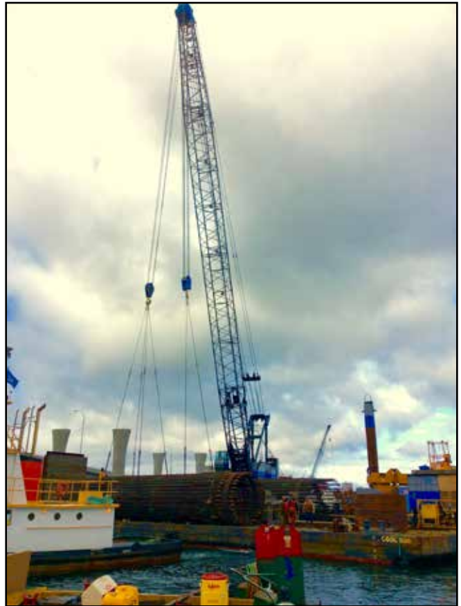
Crane Operator Chris McGrath and Oiler Todd Adams working for Pacific Pile & Marine on the SR 520 project
