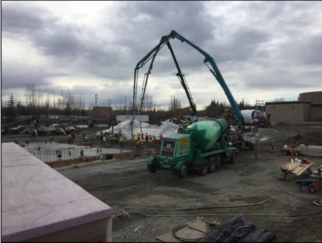
University of Alaska Power Plant
