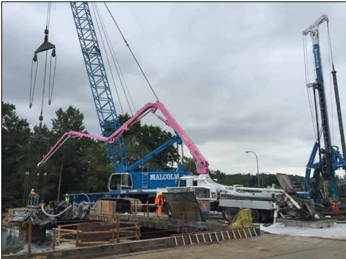
Crane Operator Kyle Wylls and Oiler Jesse Holloway working for Malcolm Drilling. Pump Truck Operator Shelby Hurley working for Ralph's on the SR 520 project.
