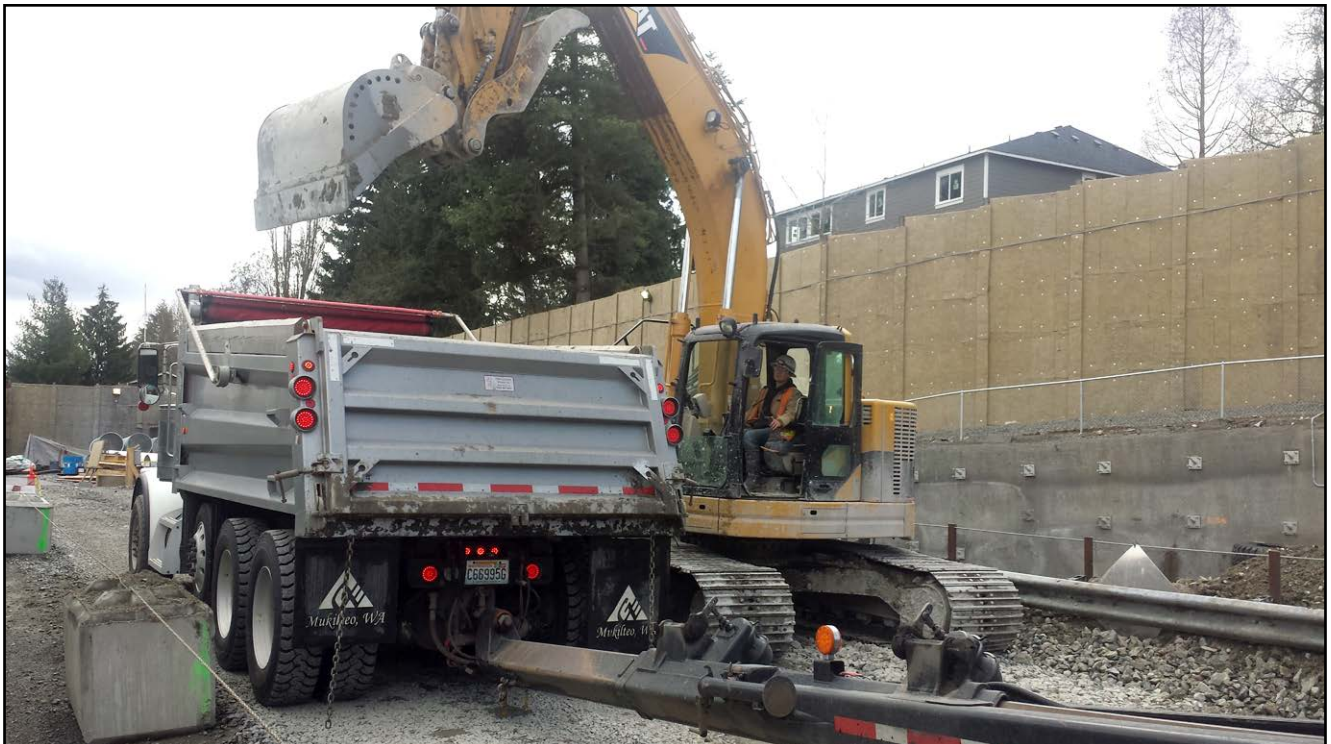
Apprentice Kim Portra loading out Trucks for Atkinson on the Sound Transit Bellevue Tunnel
