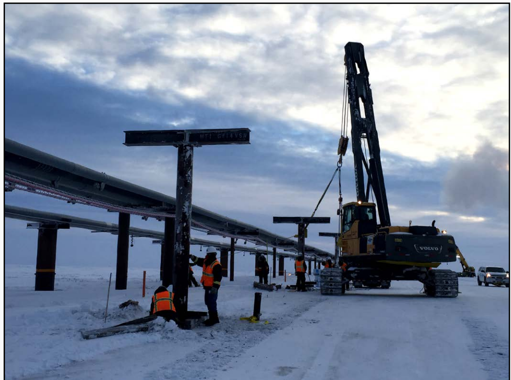
Lonnie Strickland setting VSM's on GMT-1 Pipeline Project with a Volvo Pipe Layer.
