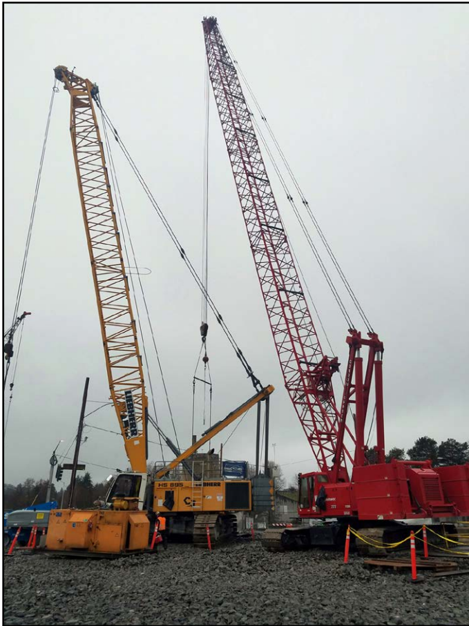
Liebherr and a 777 ran by operators Eric Seldel and Ron Nelson for Condon Johnson at the Sound Transit Northgate Station
