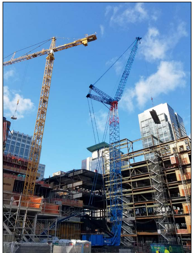
Dan Youso and Jim Wood working on the Sellen project at 9th Ave and Howell St. - Seattle WA
