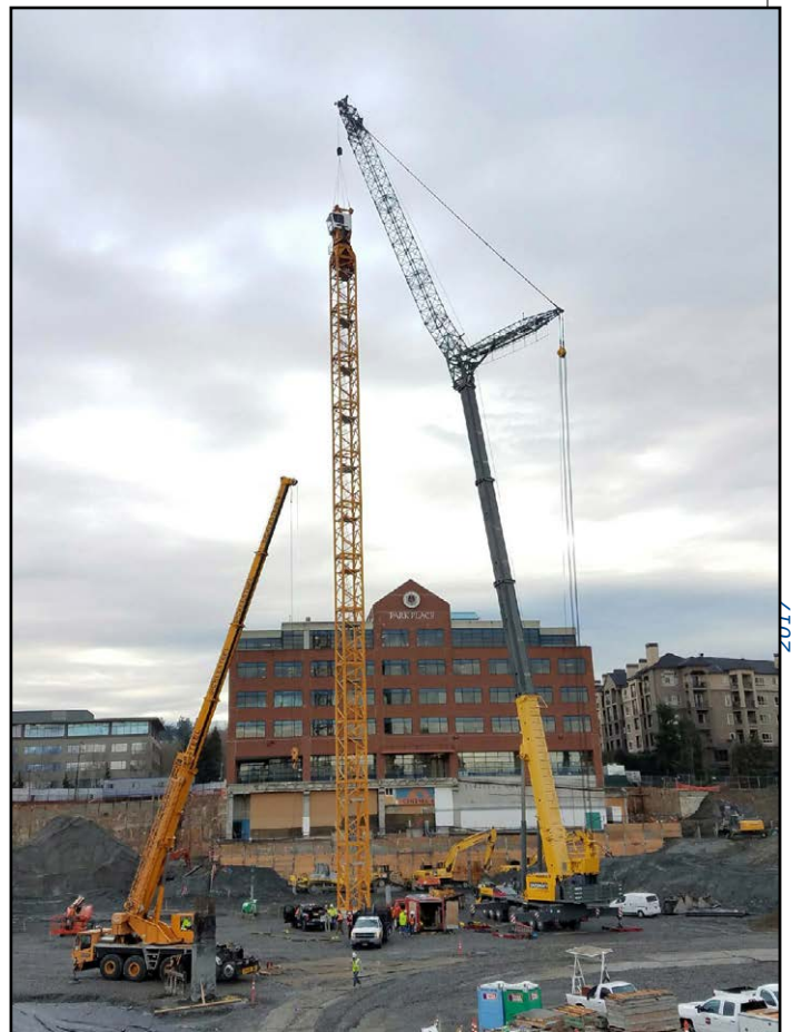
550 ton and 60 ton Erecting Tower Crane for Apex Tower Crane in Kirkland
