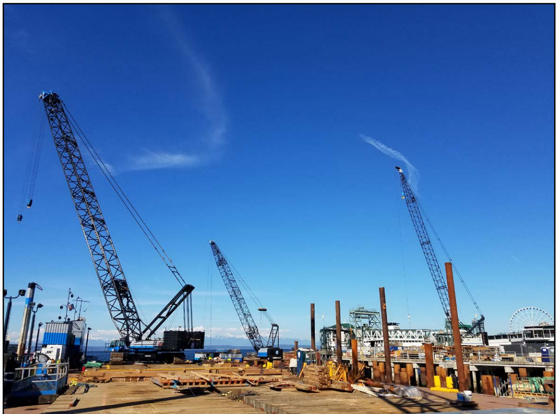
Operators Mike McLean, Mark Works, Jason Yoho, Chris McGrath, and Bruce Hyde working on the Coleman dock project in Seattle.
