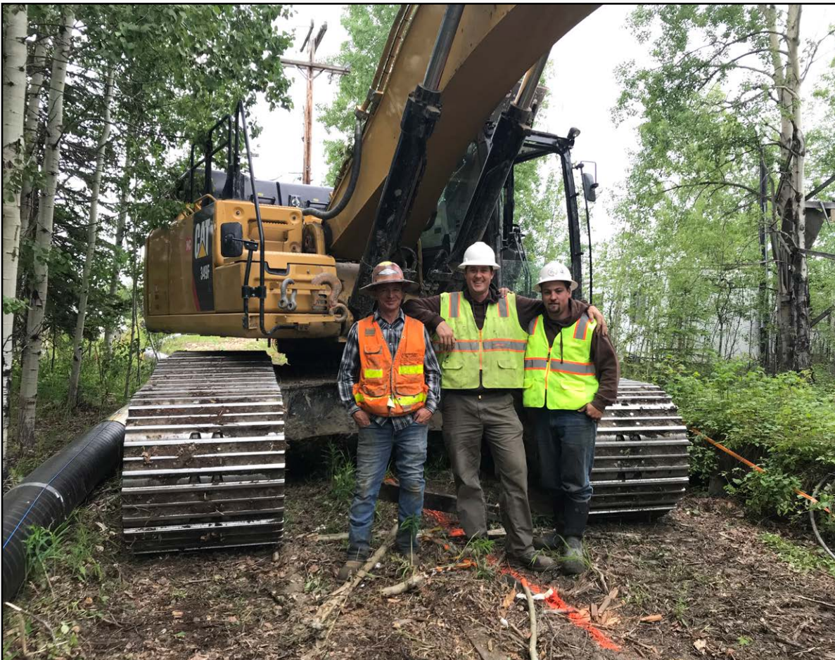
John Waddell, Matthew Himebauch, Justin Padgett - Exclusive Paving - North Pole Water Line Project
