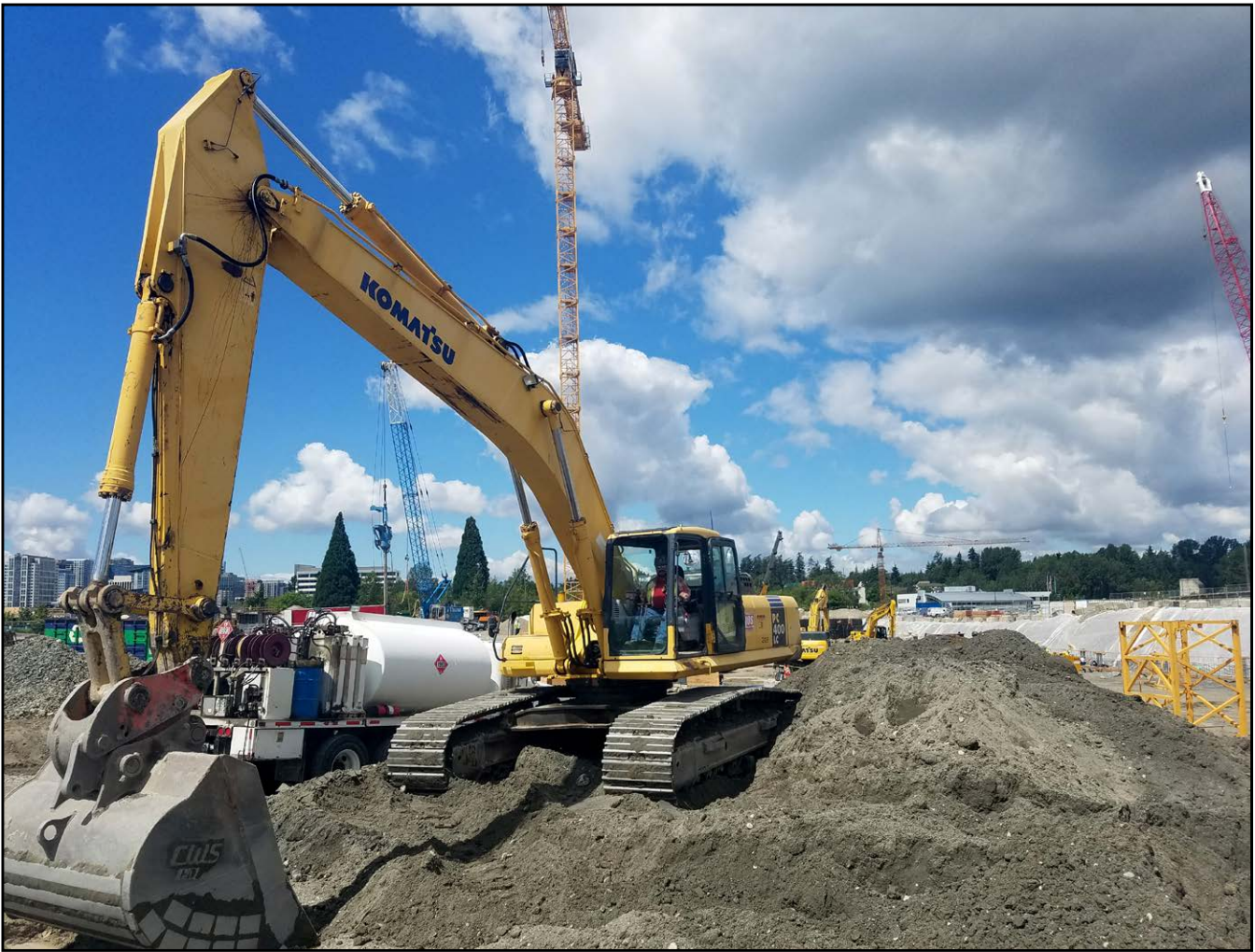
Randy Rohrer Company, Hos Brothers, Bellevue WA, REI - Project General Contractor Howard S Wright
