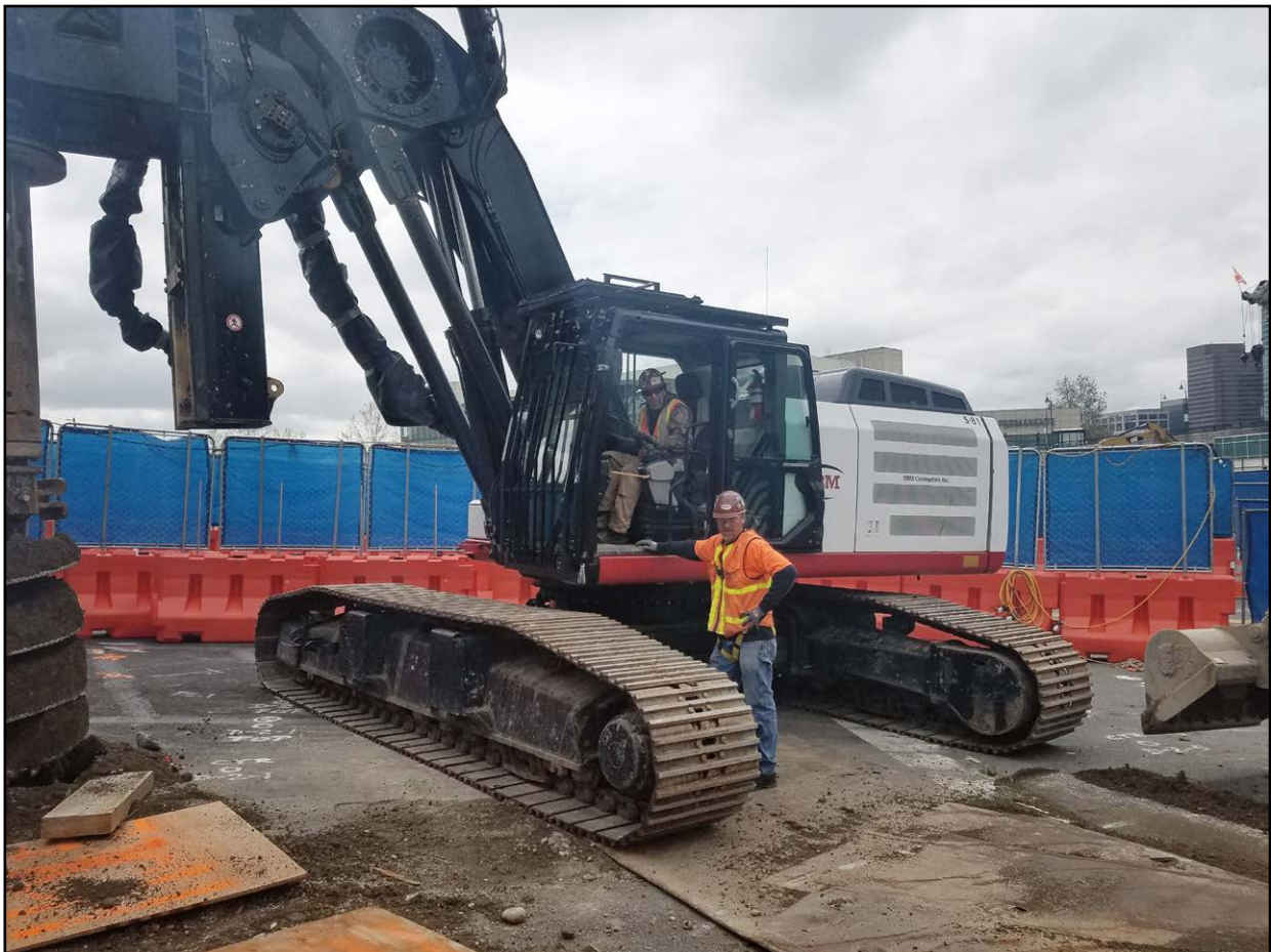
Drill Operator Terry White, Drill Oiler Jeff Sharon - DBM Bellevue, WA - Overlake Hospital
