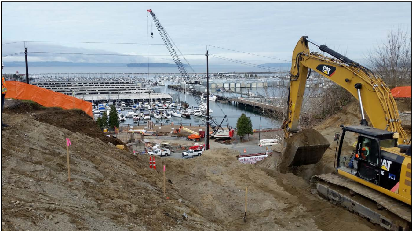
Interwest Construction Inc. Digging the upper bridge abutment for the Grand Avenue Park Pedestrian Bridge
