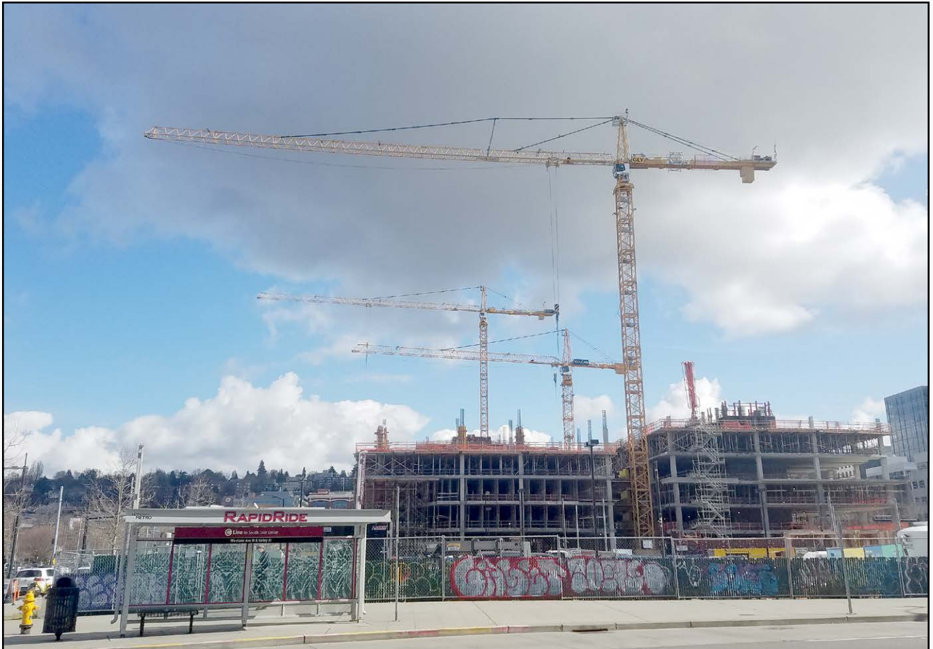
Lunch time for Operators Chance Sheridan, Mark Edwards, and Tom McFadden at GLY's Google project on south lake union.
