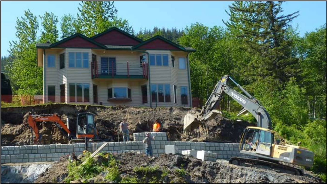
Admiralty Construction crew building a retaining wall in front of long time 302 members house Randy Beason.
