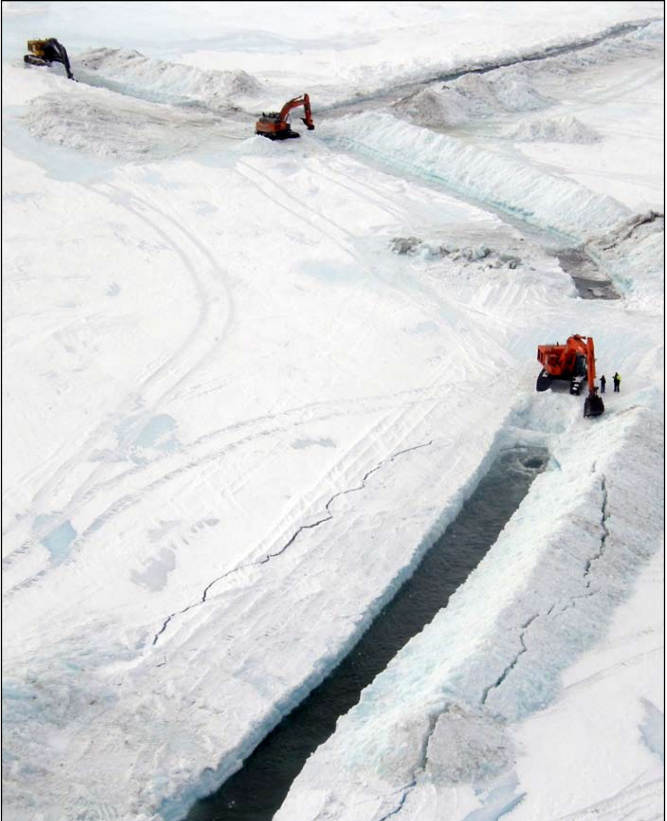
Trenching operation to restore flooded Dalton Highway. Courtesy of Ross Oliver/Alyeksa Pipeline Svc Co.
