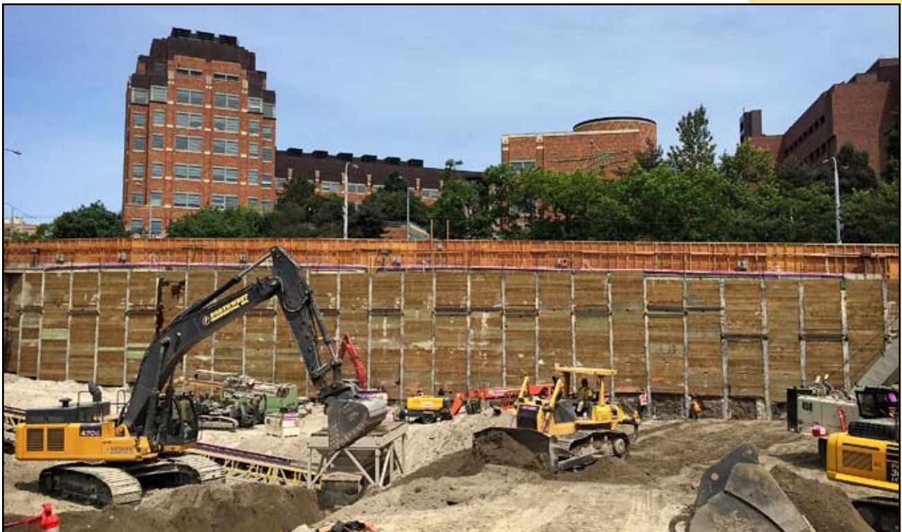
Northwest Construction and Condon-Johnson working on the Skanska ARF project at the University of Washington.
