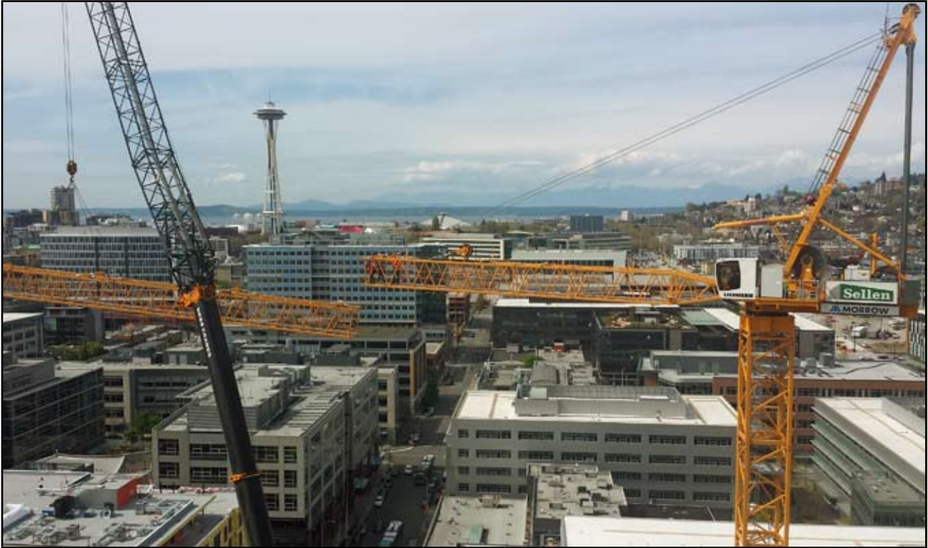
Doug Yuckert and Justin Ruth with Ness and Campbell Crane working together with Northwest Tower Crane to build Shawn Cook's Luffer he will operate for Sellen. Photo by Thomas McFadden
