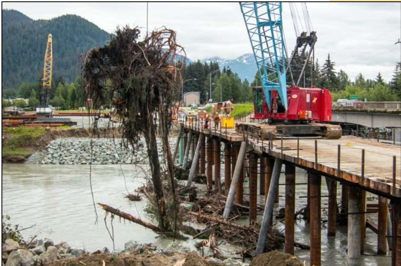
Crane operator Stacey LeProwse working for Orion Marine on the Brotherhood Bridge Project.
