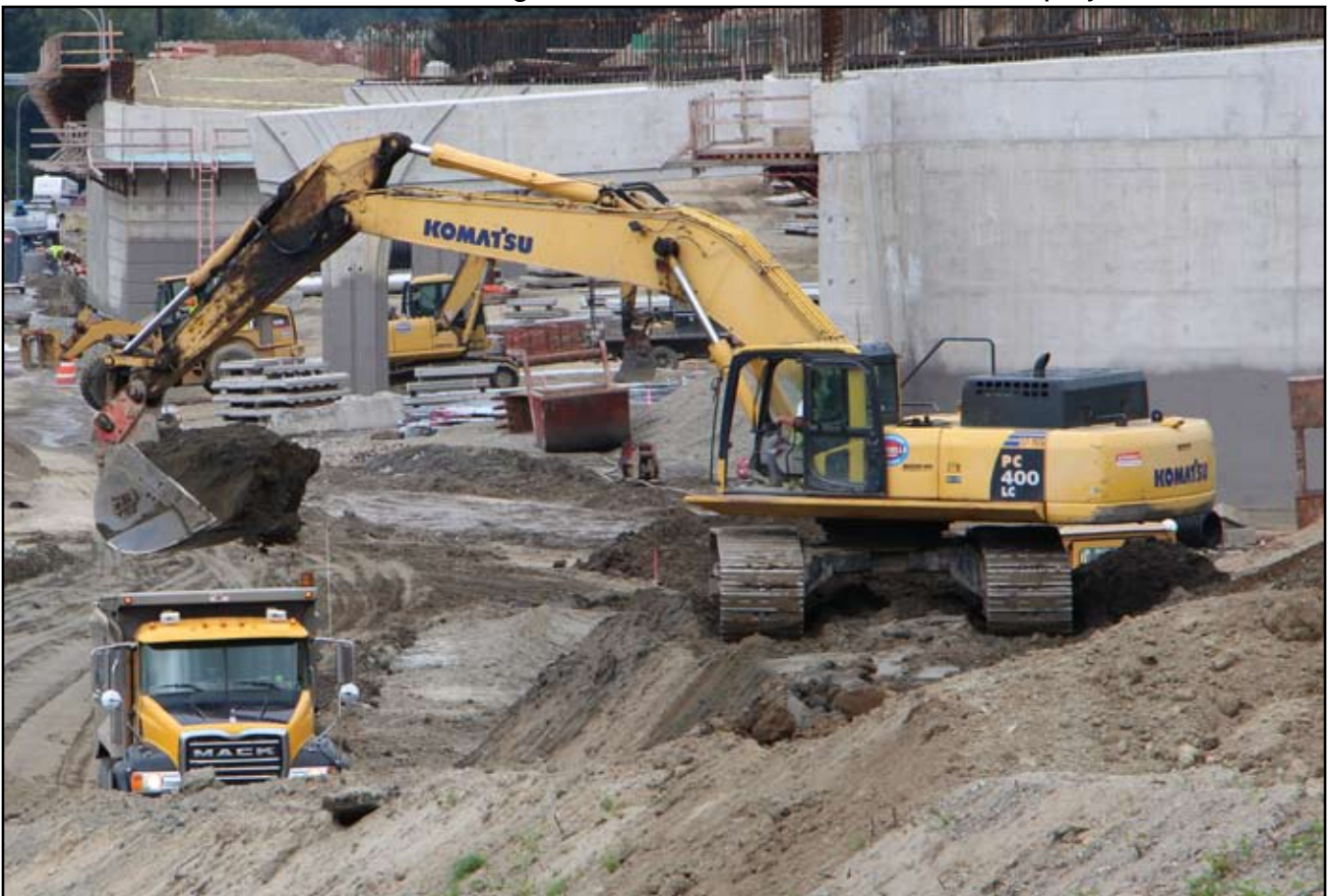
Dave Jacobs running the Excavator at the I-405 and 160th project for Scarsella.
