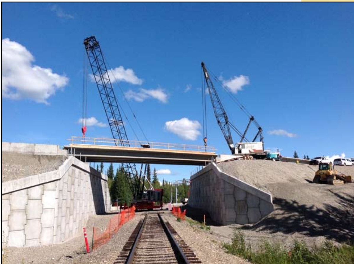
Larry Anderson and Phil Ausman setting girders on the Railroad overpass in Moose Creek
